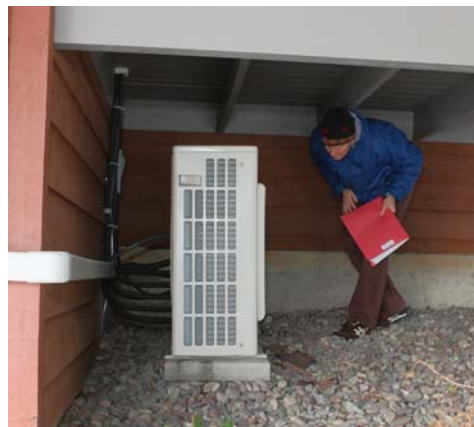
Quality Assurance Inspector Brenda Guzman inspects the evaporator/condenser outdoor unit.
