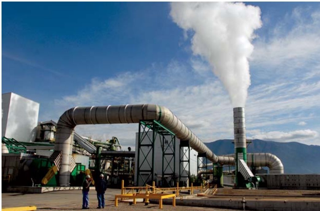
Caption: The $9.5-million biofilter at Plum Creek's medium-density fiberboard plant in Columbia Falls was unveiled at the end of October last year. - File photo by Lido Vizzutti/Flathead Beacon
